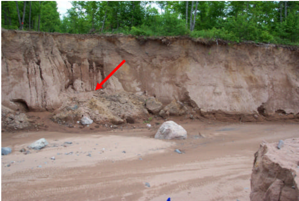
Figure 4 The upper SP-SM unit appears to contain a weak soil structure (weak carbonate cementation?) that when disturbed loses strength and crumbles (pile at arrow). This unit has a low dry strength and is easily broken by light finger pressure. View is of left channel downstream of former fuse plug.
