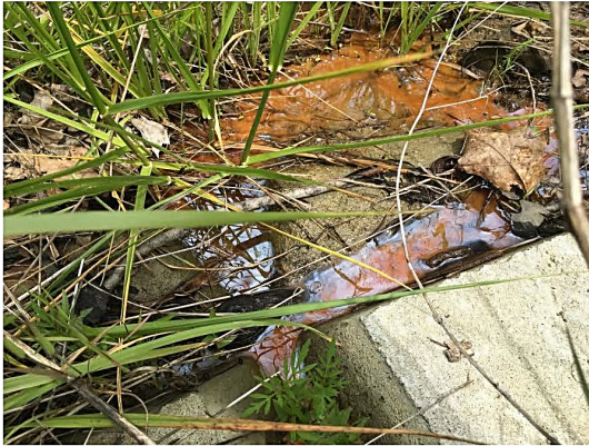
Oily sheen of the water is concerning... is there a leak?
