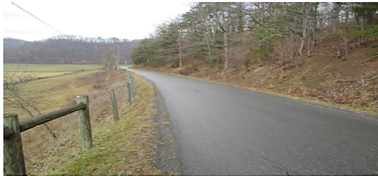
Hans Creek Road slid away in 1975 at this point, according to Google Earth it is located at 37.547616, -80.725168
