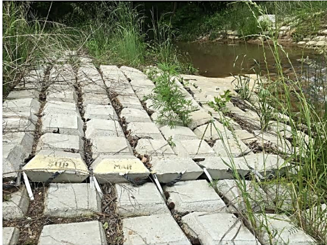
The concrete mesh spans the easement ROW covering the creek with concrete.
