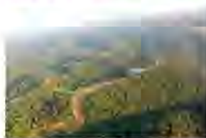
Cross-country pipe being installed. ©Ed Wade, Wetzel County Action Group, FracTracker Alliance
