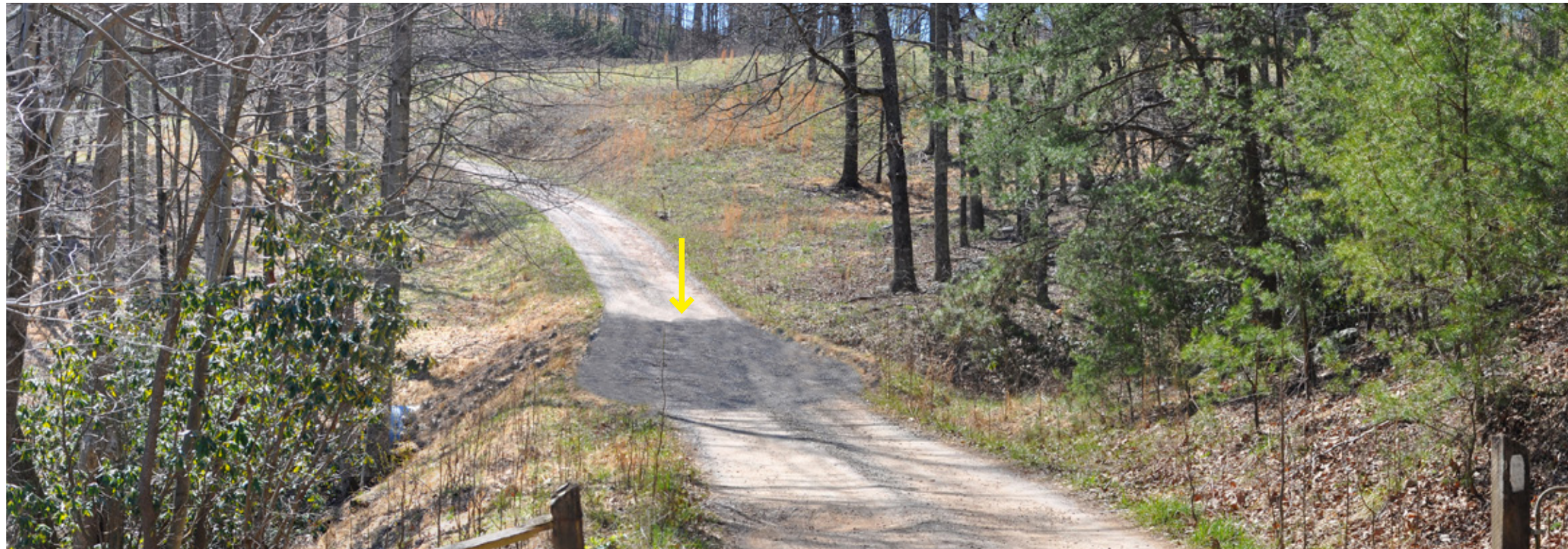
Post Construction (Leaf-off conditions) - From this location modifications to the roadway would be apparent where culvert upgrades would occur. The yellow arrow indicates the modifications to the roadway.
