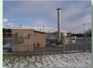
Metering and Regulating Station
