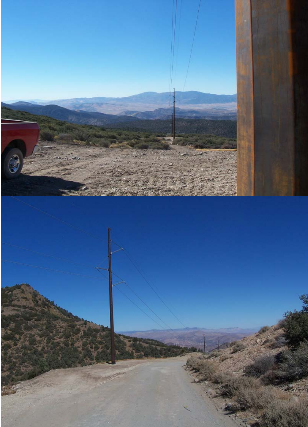
Figure 3-19. Photograph of an existing single circuit steel mono-pole transmission line similar to the one proposed for the Swan Lake North Hydroelectric Project (Source: Electrical Consultants Inc. 2019)
