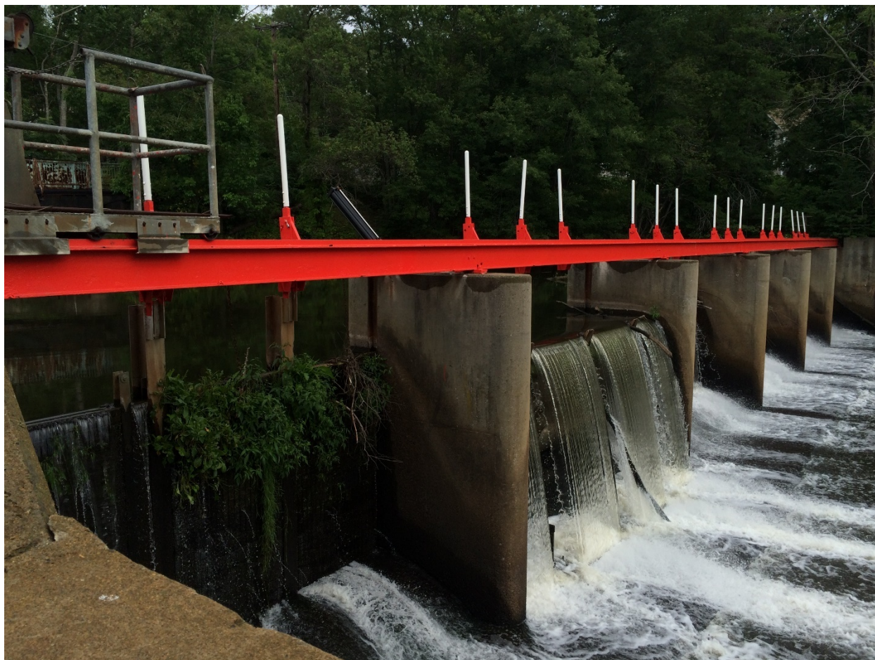
Figure 3. Photograph of the Riverdale Mills Project dam. (Source: Blackstone Heritage Corridor, undated).
